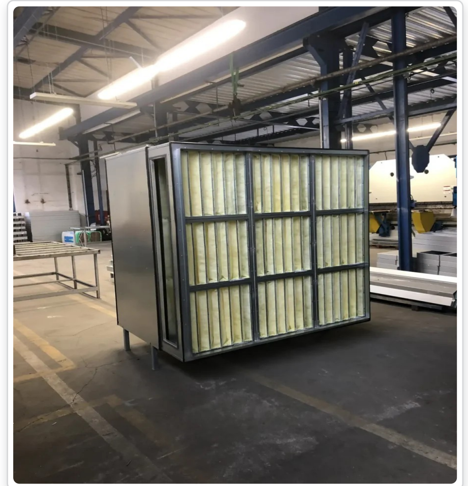
Multi-stage filter unit for an industrial intake silencer
